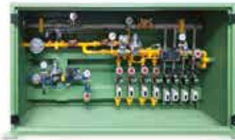
Oxy-Fuel Kontrol Hattı Oxy-Fuel Control Line
